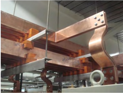
Transformer lead to Terminal
