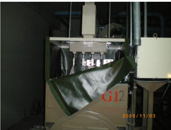
Generator lead to Terminal
